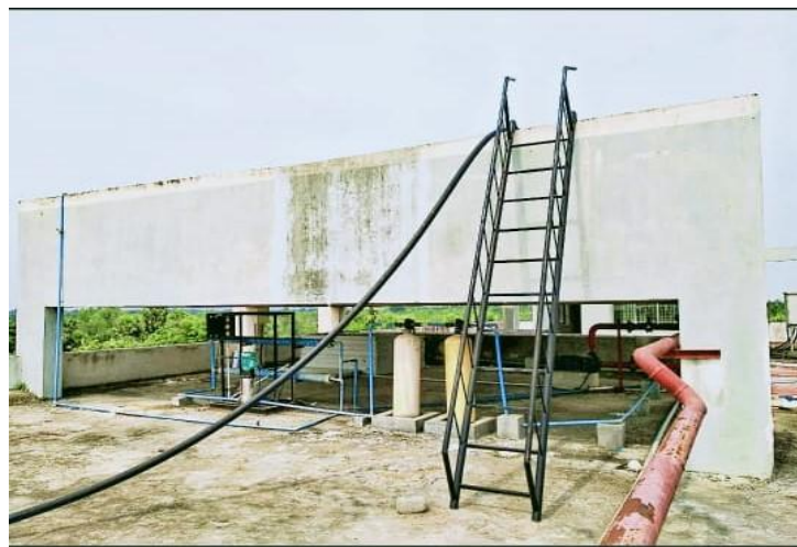
Figure 2: Overhead Water tank
