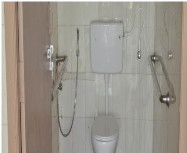
Physical facilities for differently abled – (4) Toilet with hand rails
