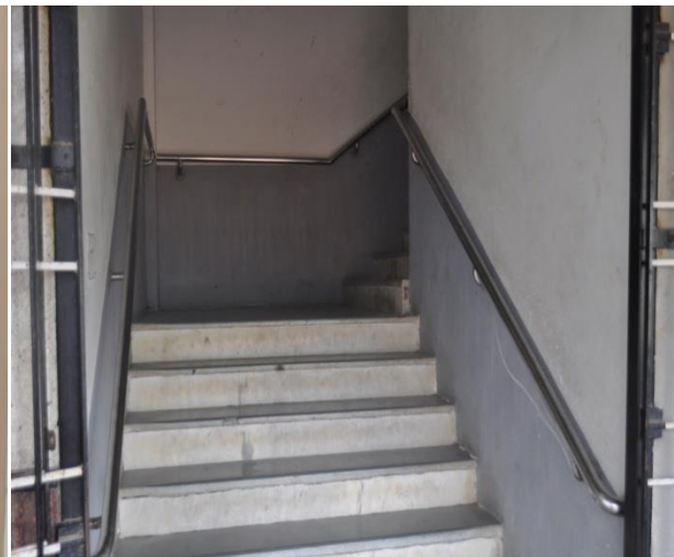
Physical facilities for differently abled – (5) Foot step with hand rails
